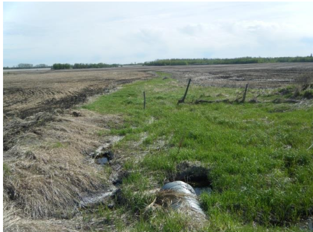
Photo 43: Ephemeral pathway permitting water movement to Wetland 8 (facing NE). Note culvert connecting water to pond in Photo 42.
